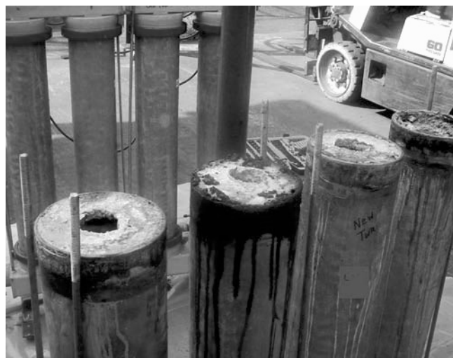
Figure 3 8 inch cells used to treat 450 ton industrial cooling tower under zero discharge mandate.
